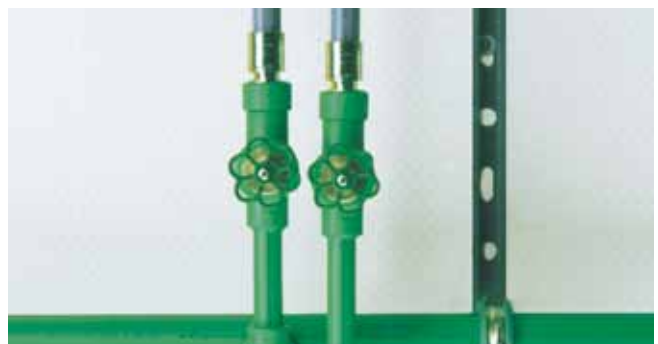
aquatherm grey pipe connection
