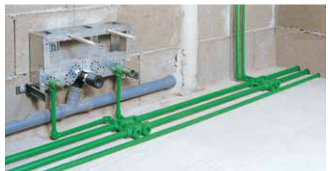
Floor distribution with distribution blocks
